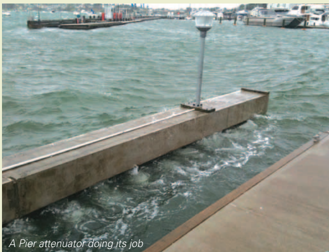
Piles? What piles?
